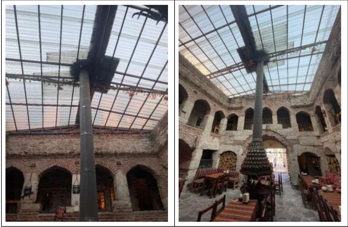
Figure 8. Examples of deterioration observed in Aşağı Taşhan
