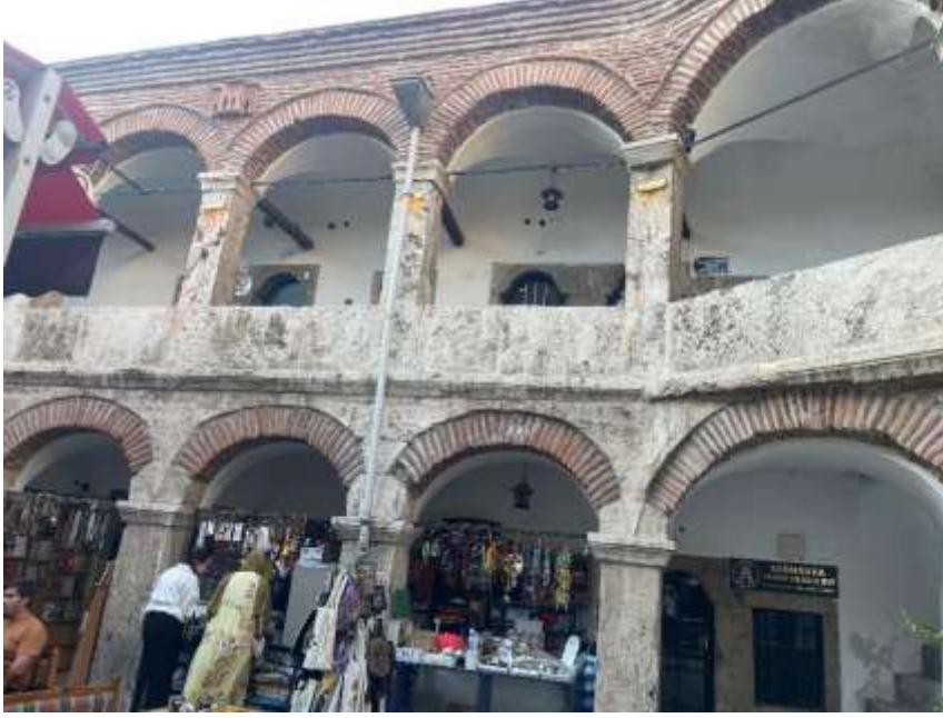
Figure 3. Examples of surface deterioration on the building
